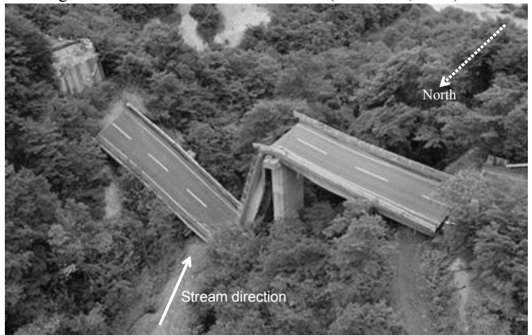
Photo. 1. Collapse of the Maturube Bridge.
