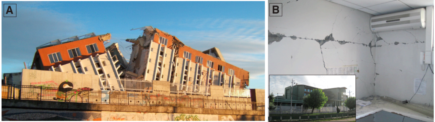
Fig. 2: (A) Collapsed 20-story apartment complex located in downtown Concepción near the Bío Bío River. (B) Damage to newly built (2008) hospital facilities in Curanilahue (near Arauco) about 80 km southwest of Concepción. The hospital sits on an old river channel and evidence of liquefaction was observed following the earthquake. Estimated ground motion for such coastal sites of NEHRP soil class D (stiff soil) equivalent is 0.4g (GEER, 2010) (photos by C. Neighbors)
